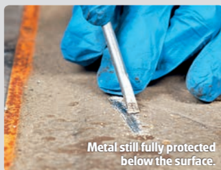
Rusty wax in the seam. Metal surface of the seam showing signs of corrosion.
