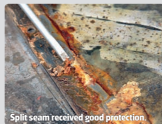
Split seam received good protection.
