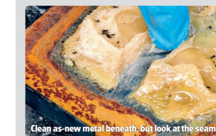
Clean as-new metal beneath, but look at the seam.
